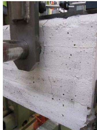
Figure 5. Photo taken before testing, at the end where failure later took place. Second test specimen, low corrosion
