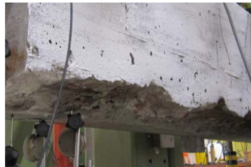
Figure 6. Photo taken before testing, at the end where failure later took place. Third test specimen, high corrosion with cover spalling.
