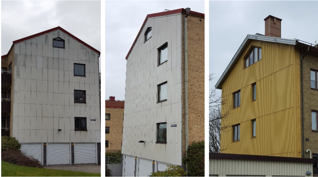
Figure 7. Often the south façade is renovated. Examples of two different strategies where cementitious boards (left) and a metal cladding (right) were chosen on the south facade.
