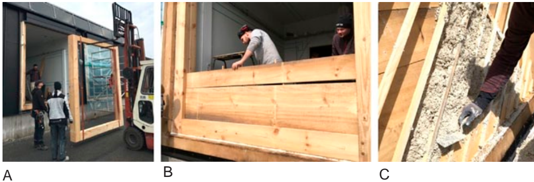
Figure 5. Construction of two full-scale test walls at Lund University, A) Construction of post-and-plank walls, B) Timber planks mounted between the posts, C) Application of hemp-lime on the post-and-plank wall. Photos: Paulien Strandberg.
