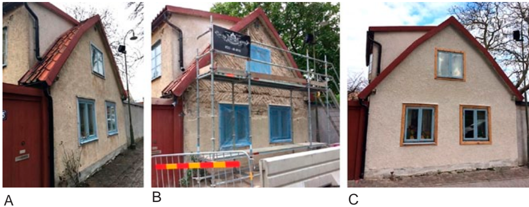
Figure 4. Detached historic single family house in Visby renovated with hemp-lime, A) Before renovation, B) During renovation, C) After renovation. Photos: Paulien Strandberg.
