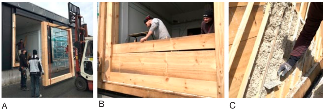
Figure 5. Construction of two full-scale test walls at Lund University, A) Construction of post-and-plank walls, B) Timber planks mounted between the posts, C) Application of hemp-lime on the post-and-plank wall. Photos: Paulien Strandberg.
