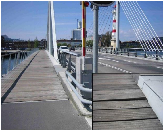
Figure 7. Deterioration of the wooden planks on sidewalks of the university bridge, Photo courtesy of Per Andersson
