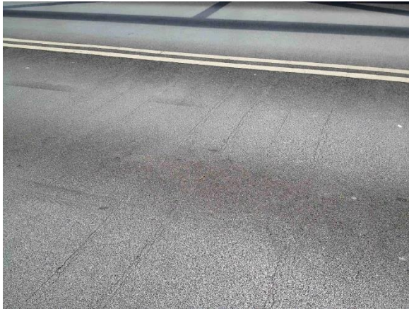
Figure 3. Wear of the surface and transverse cracks in the orthotropic steel deck, Photo courtesy of Per Andersson
