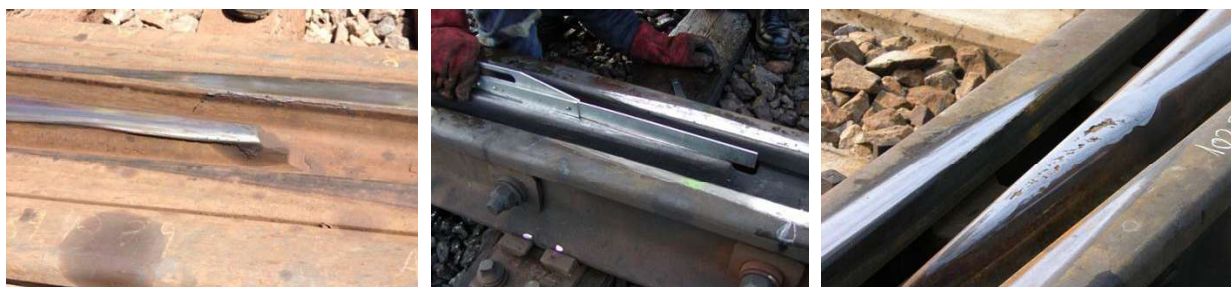
(a) Plastic deformation (b) Wear (c) Rolling contact fatigue
