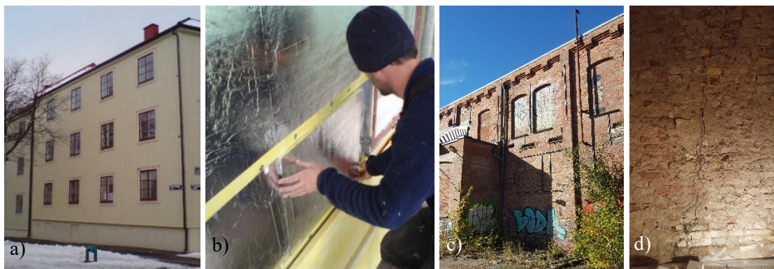
Figure 1. Installation of insulation on the interior or exterior of listed buildings. a) Multi-family building from 1930s in Gothenburg [12], b) Installation of VIPs on the exterior, c) Industrial building from 1896 in the south of Gothenburg, d) Sensors inside the case study building.
