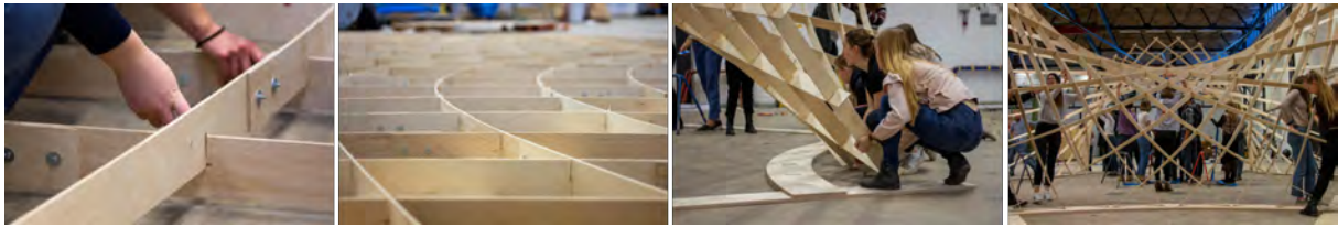
Figure 8: a) connecting the laths into a flat grid shown in b). c) - d) the structure was erected by pushing the structure with manual force, photo: Brobäck, Ivarsson & Skarby. [14]
