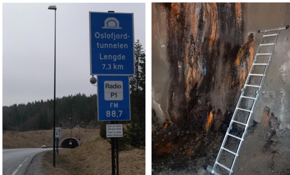
Figure 7. The Oslofjord tunnel entrance (left) and microbial biofilm material on sprayed concrete on the tunnel wall (right).
