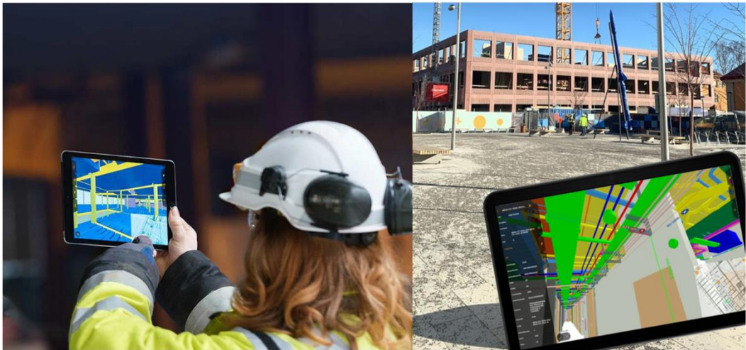
Fig. 3: Left: Use of StreamBIM on-site. Right: View of the Celsius project during construction
