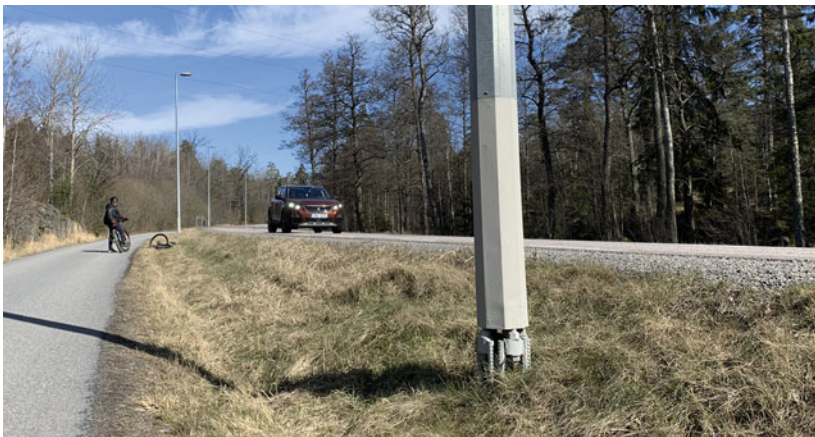
Fig. 16 Lightning column with a deformable element in the base aimed to lower vehicle acceleration in a crash. (Photo: Helena Stigson)
