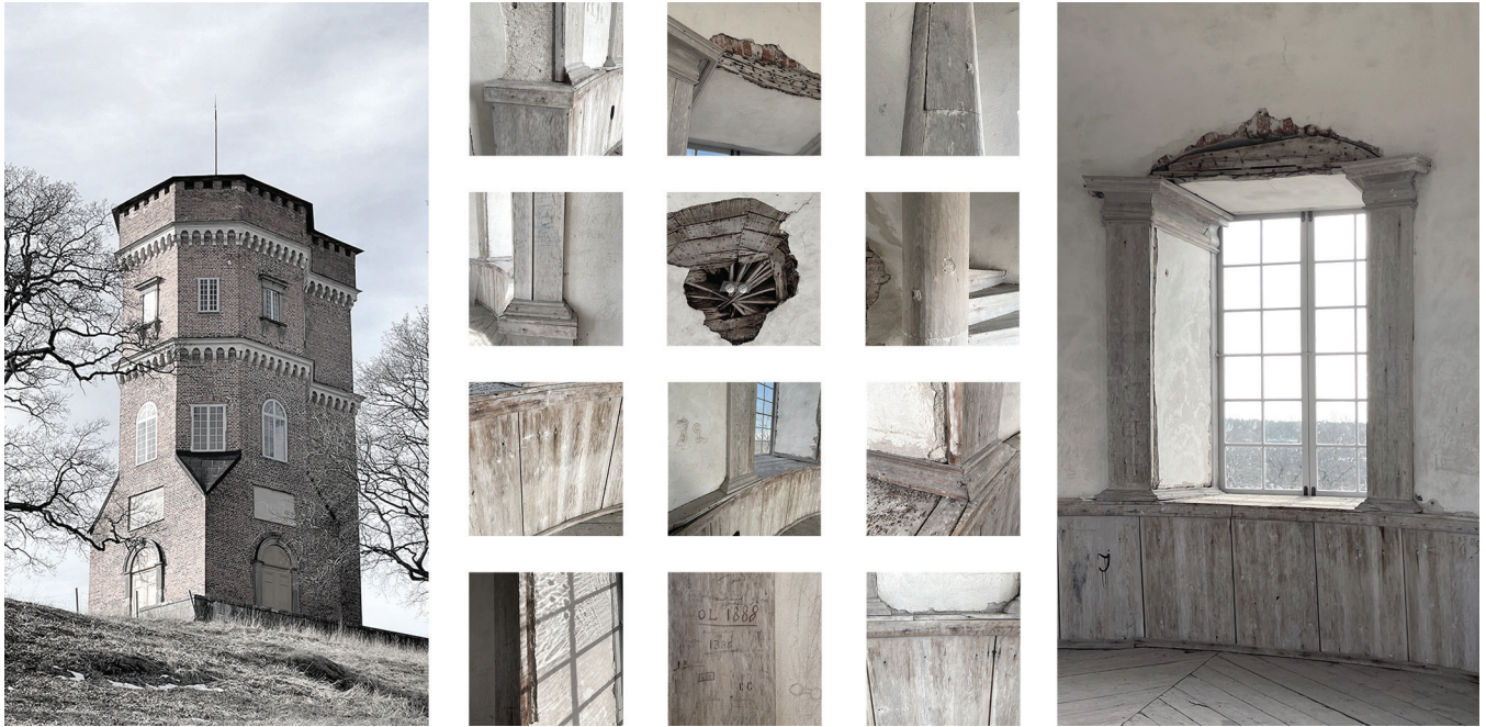
3 Eighteenth-century tower 'Götiska tornet' in Stockholm, Sweden (left), with an inventory of deteriorated wooden elements (middle) and an incomplete wooden window casing selected for the experimental restorative intervention (right).
