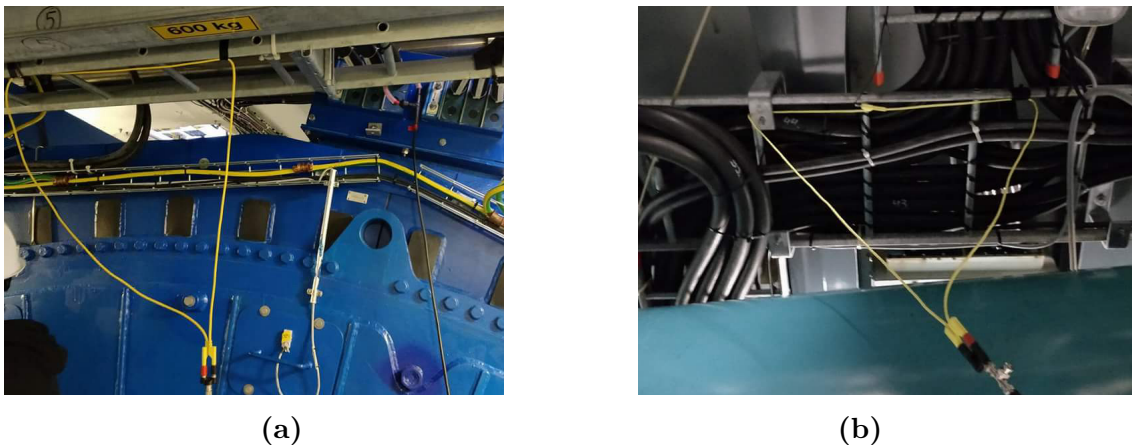
Figure 3.4: The voltage measurement loops at Big Glenn site (a) near the generator (b) above the shaft
