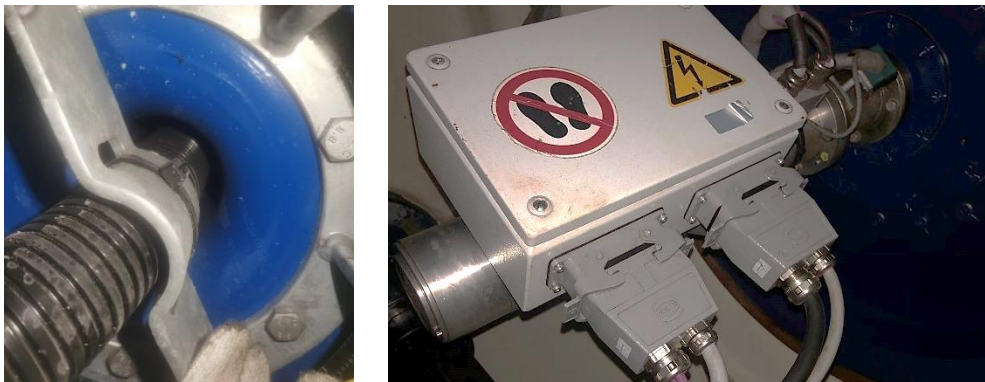
Figure 3.7: Hub power cable through hollow shaft hub side view and nacelle side view with the slipring connection box.
