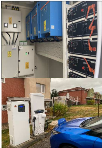
Fig. 5. Stationary battery (left) and V2G charger (right)
