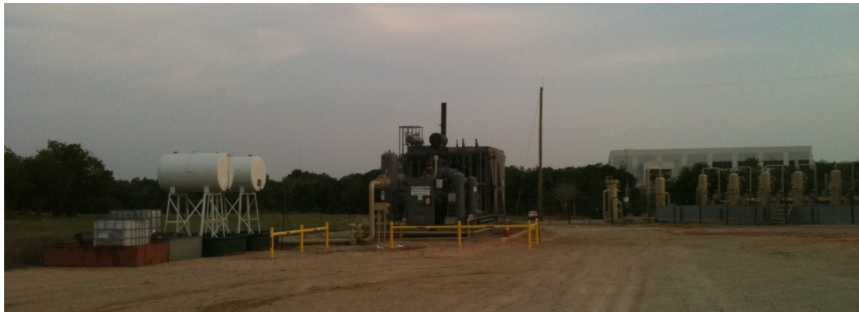
Figure 84 The compressor and separators near Meacham Blvd.
