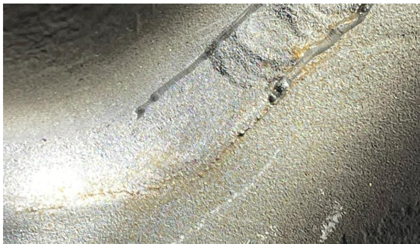
Figure 10: HFMI-treatment revealing shallow, sub-surface porosity. Also visible are surface (possibly cold) cracks at weld toe. Such weld should be repaired prior to HFMI-treatment.
