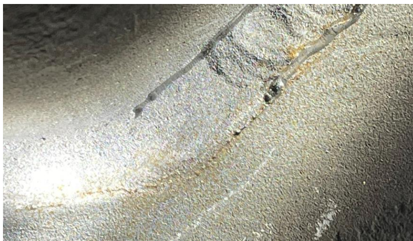
Figure 10: HFMI treatment revealing shallow, sub-surface porosity. Also visible are surface (possibly cold) cracks at weld toe. Such weld should be repaired and re-treated.
