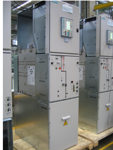
Fig. 1. A typical electric switchboard (Wikimedia, https://commons.wikimedia.org/wiki/File:Medium_voltage_panel.jpg ; Retrieved 05/01/2021)
