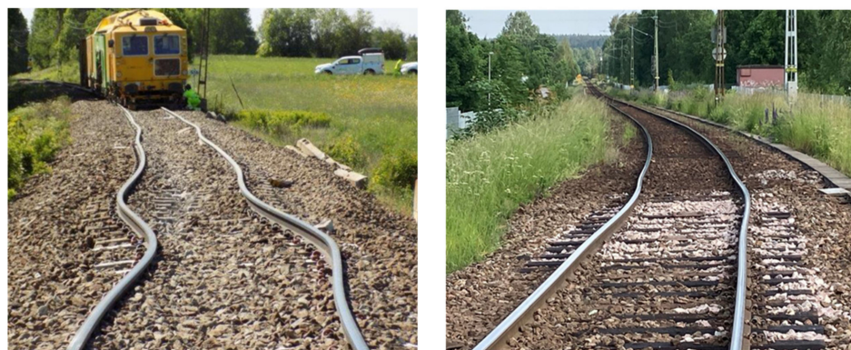
Figure 1. (Left) Lateral track buckling related to continuously welded rail on concrete sleepers in summer 2020, and (right) lateral track buckling related to continuously welded rail on timber sleepers in summer 2021 (photos provided by STA).
