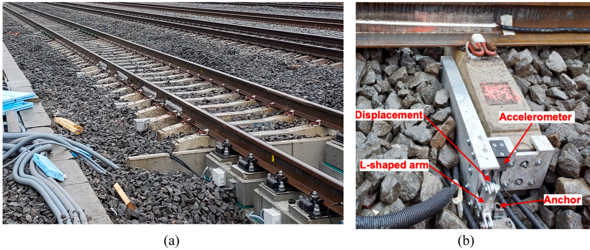
Fig. 16. (a) Overview of the transition zone between the ballasted track and 3 MB slab track at Gransjö, Sweden. (b) Detail of an instrumented sleeper equipped with a vertical base plate, an L-shaped mechanism, one accelerometer and one displacement transducer. The positions of the anchor tip and the L-shaped mechanism with a swivel and a roller are shown [20].
