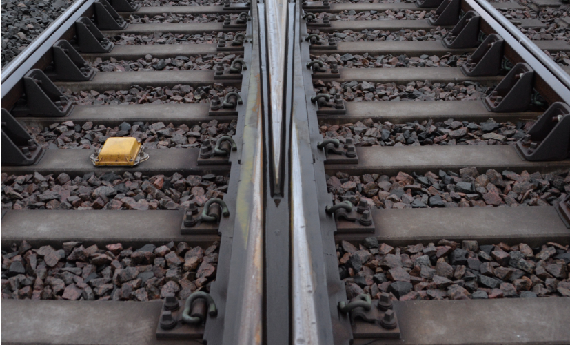
Figure 2.2: A crossing rail (two wing rails and a crossing nose) within a crossing panel.
