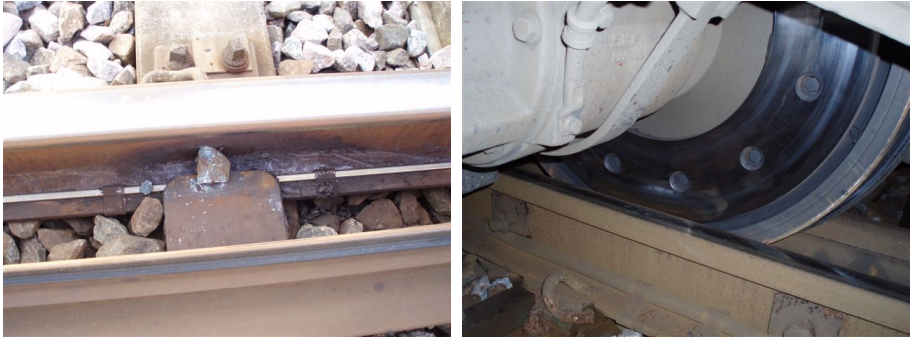
(a) Ballast stone on a sliding chair leading to (b) Flange penetration between switch and stock rail due to ballast stone gap between switch and stock rail
