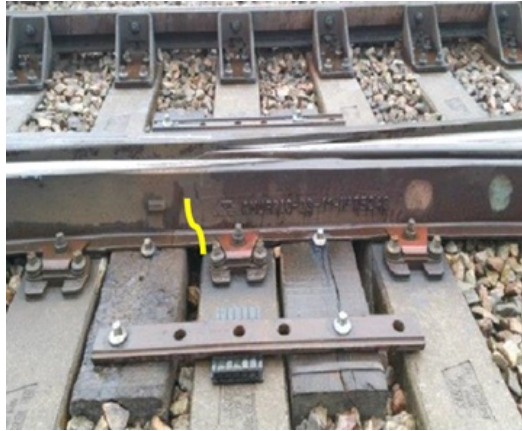
Figure 65-1 Common crossing cracked in the foot flange area (crack in yellow)
