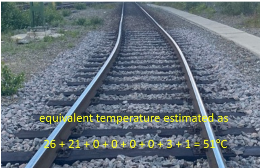
Figure 24-1 Track buckle with corresponding evaluation of equivalent temperature as a sum of contributing factors. Picture Trafikverket.
