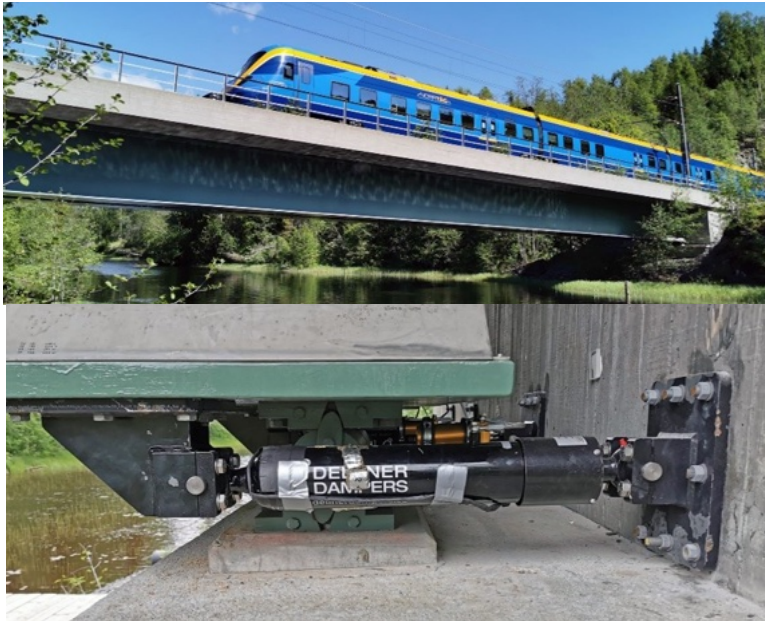
Figure 68-1 Top: view of the bridge during passage of an X62 train, bottom: details of the retrofitted damper near the roller support.
