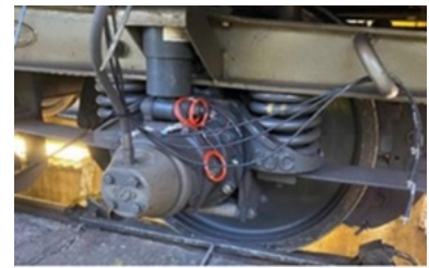
Figure 71-1 The installed ABA system
