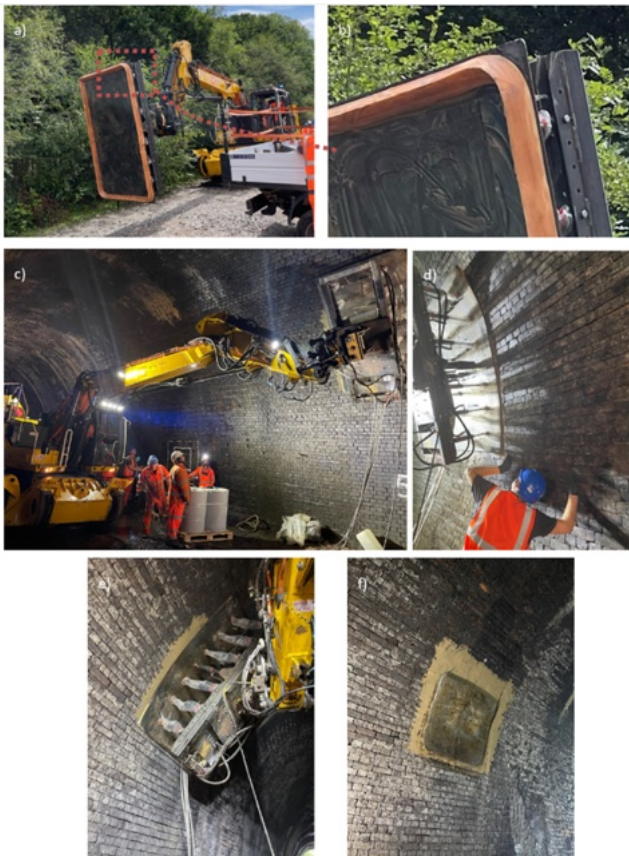
Figure 74-2 The flexible plate for the demonstrator (a), detail of perimeter seal, (b) execution of the repair (c, d and e) and patch repair after removing flexible plate
