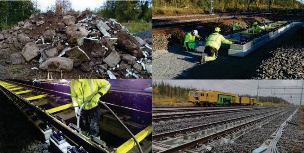
Figure 62-3 Large boulders found during excavation (upper left), whole modules being positioned (upper right), pouring of levelling mortar (bottom left), finished track section at 96 hours (bottom right).
