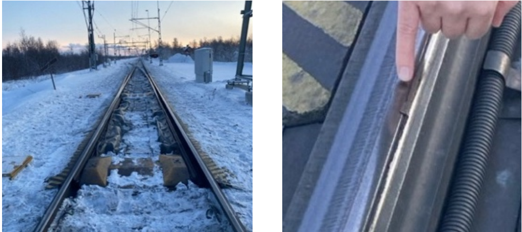
Figure 30-1 Left: Switch & crossing at the Iron Ore line. Right: Plastic deformation of the tip of the switch rail.
