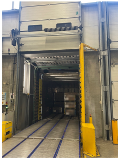
The pallets loaded onto the trailer. Matching conveyors are installed in the trailer
