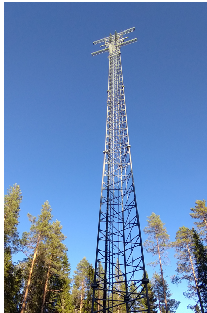
(b) BorealScat-2 radar tower.
