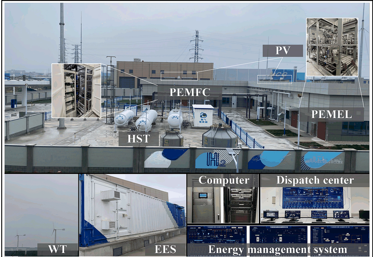
Fig. 10. Hydrogen-electric coupled DC microgrid demonstration project.
