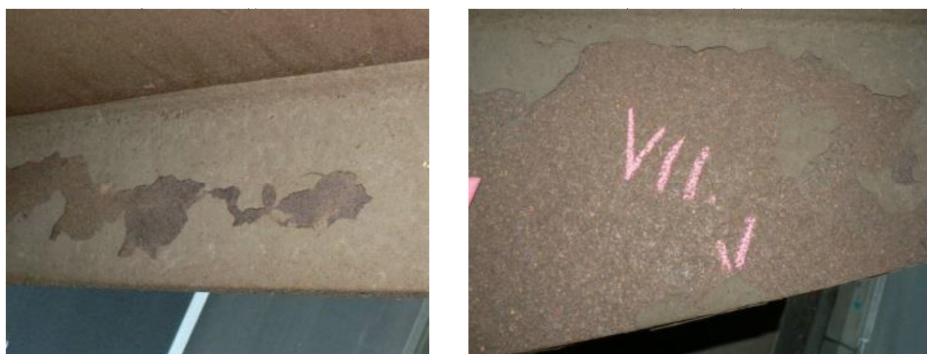
Non adherent rust layers
