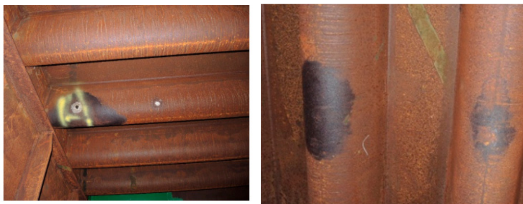
Figure 4. Drainage leakage effects (Reprinted from Ref. [42]).
