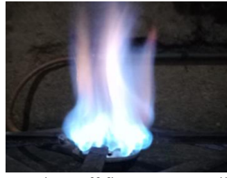
(d) Blow-off flame, many yellow zones, safety-risk indicating high pressure due to underutilisation, unreleased vapour and potential impurities.
