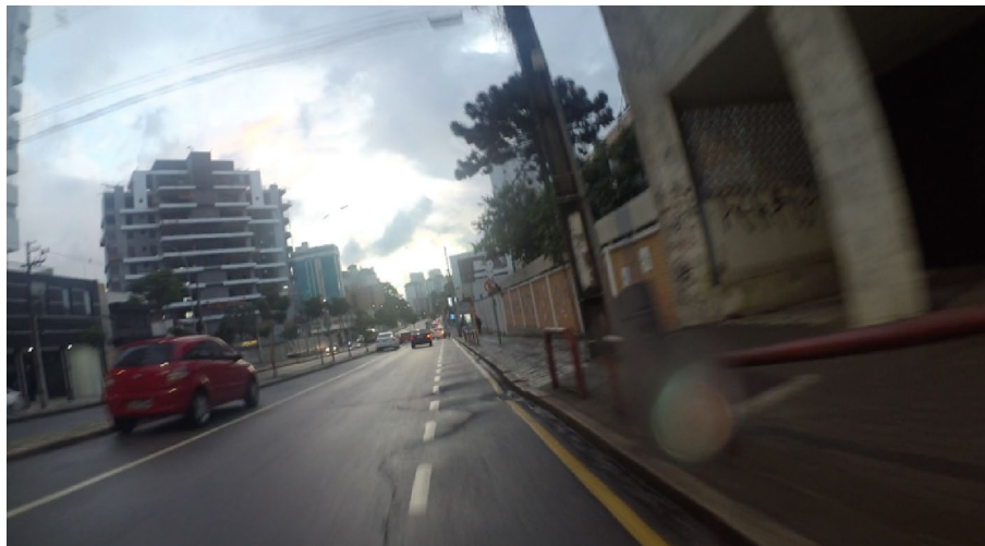
Fig. 15 Cycling lane in Curitiba with a defect in the asphalt on the bicycle area of ride
