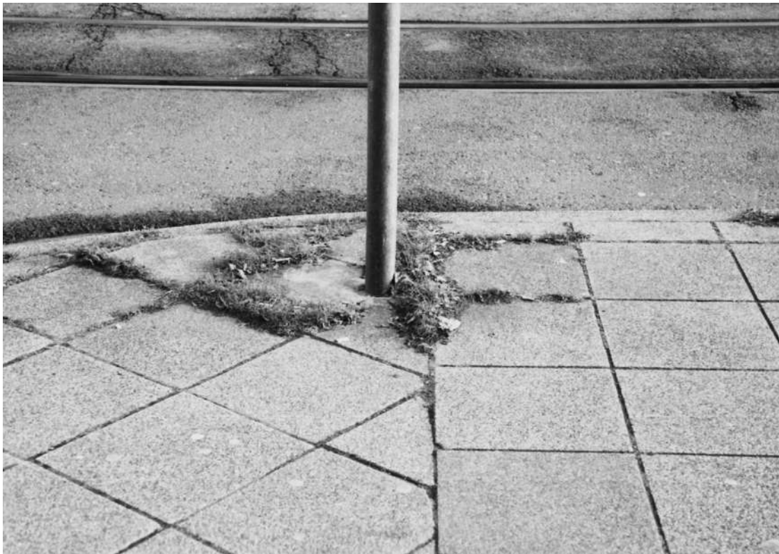
Fig. 2: Image of excessive pavement in Ghent, Belgium, where soil species can only sporadically break through cracks.
